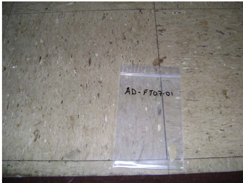
Photo 2 – View of brown floor tile containing 4% Chrysotile.
