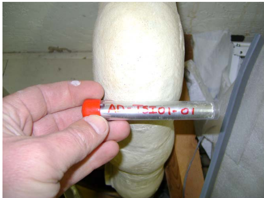
Photo 6 – View of hard-packed pipe fittings containing 8% Chrysotile.
